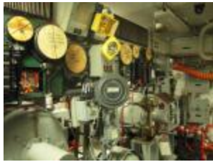
Starboard Steering Gear Power & Control Room
